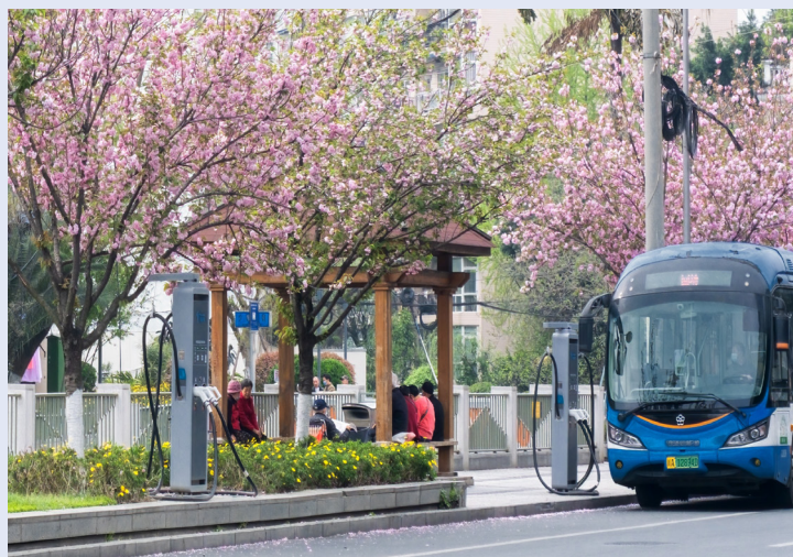
Battery charging stations for electric buses on a road in Chengdu, Sichuan. SOURCE: B. Zhou via Shutterstock
