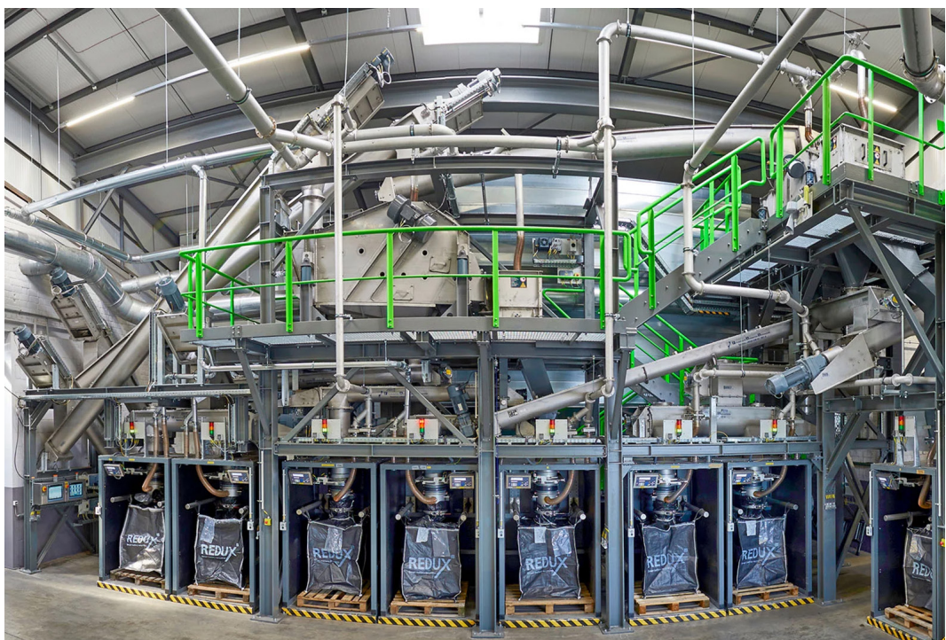
Battery recycling plant. SOURCE: Saubermacher
